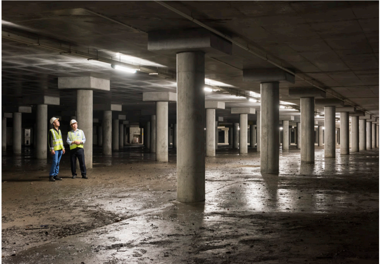
地下蓄洪池容量達6萬立方米 Underground stormwater storage tank with a capacity of 60,000 m 3
