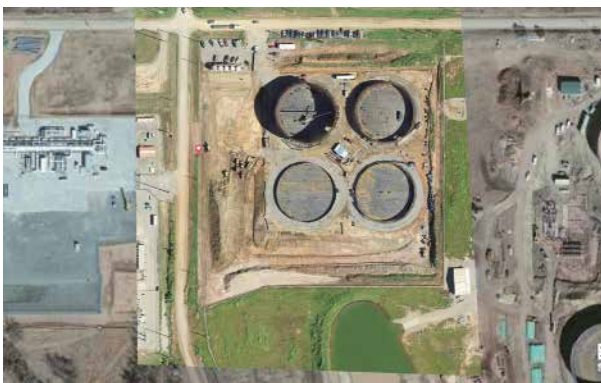
The same construction site orthomosaic map is re-rendered as a Digital Surface Model (DSM), allowing for the easy measurement and extraction of area and volumetric of excavations and materials on site.
