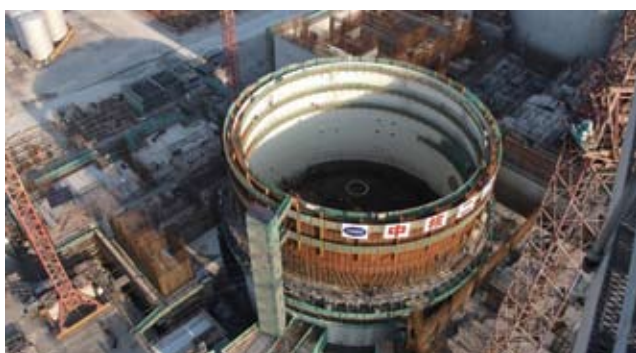
AP1000 NUCLEAR PLANT AT SANMEN (CHINA). CRESCO-GROUP DESIGNED THE FINAL ENGINEERING OF SEVERAL INTERNAL STEEL STRUCTURES AND OF THE CONICAL ROOF FOR ANSALDO NUCLEARE
